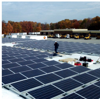
500 kW commercial system
